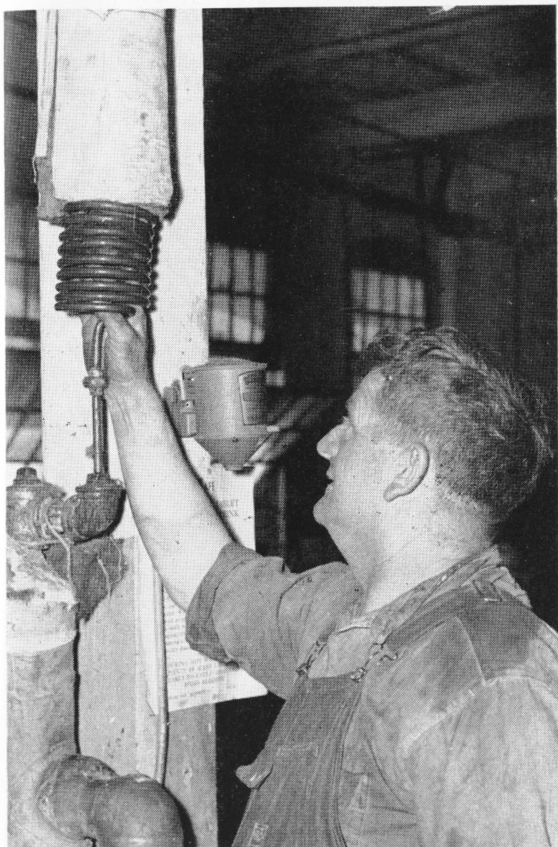
To make sure all the bubbler fountains get the same pressure of water, and to keep it from playing tricks on you by dying down and spurting up just at the wrong time, circulating balance coils like these are installed all over the place.
